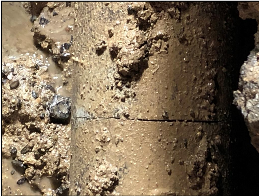
Broken 6" AC main line
