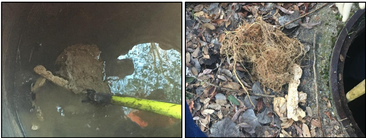
Root ball and grease broken lose from Hydro Flushing left Root ball and grease removed right
