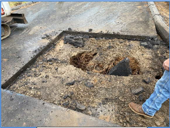
Sink hole under asphalt due to broken service line
