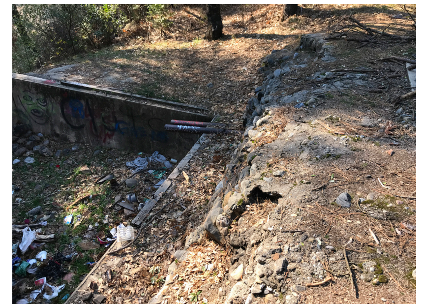
Improved safety - remove debris or old and obsolete infrastructure.
